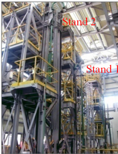
Fig.1. The HBM setup consists of 2 stands, and both of them can be operated independently to execute slag modification.
